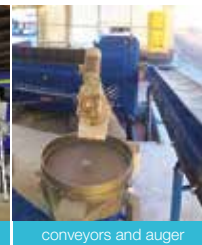
conveyors and auger
